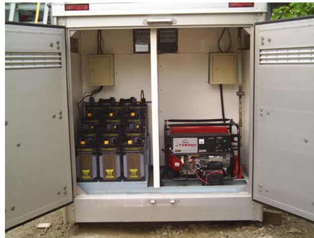
Figure 9. Battery room and Diesel room
