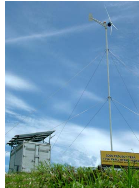
Figure 2. 1 kVA-Hybrid Power Plant
